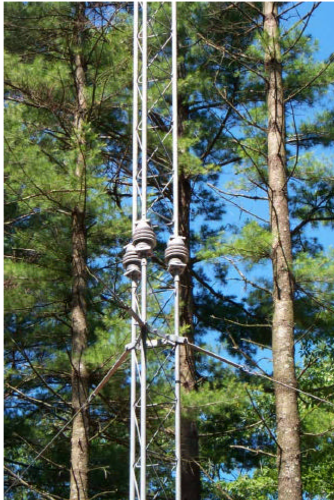
Photo 2: Tower leg insulators at elevated radial feedpoint (photo by WIFV)
